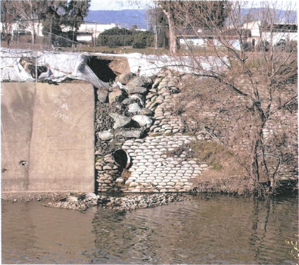
Failing Outfall 138 along Los Gatos Creek adjacent to County Park
