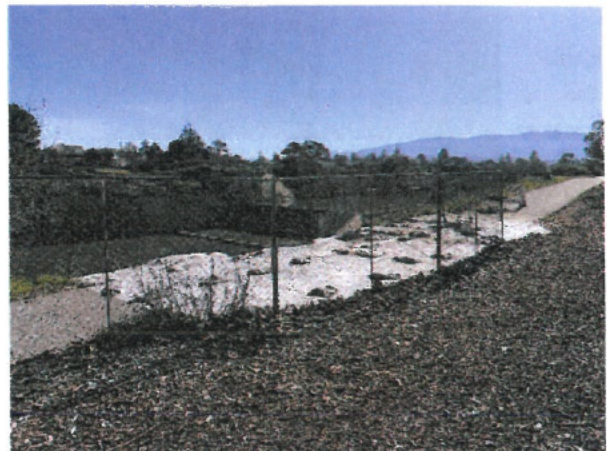
Fencing around sinkhole - failing outfall
