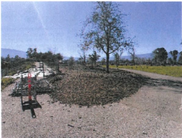
Los Gatos Creek County Park pathway closed due to failing outfall
