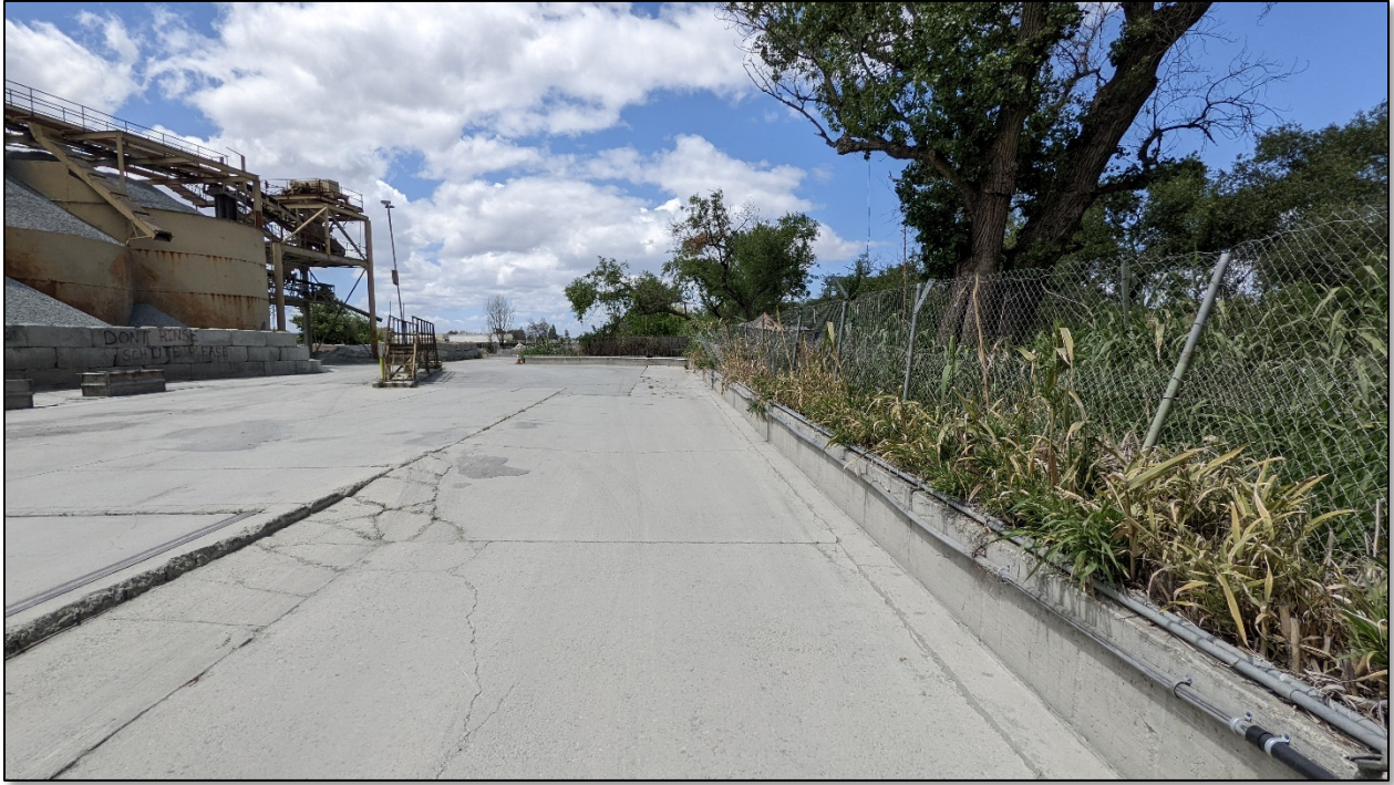
View of TCE 378 located to the west of the utility building, as seen from along the northeastern boundary, facing northwest
