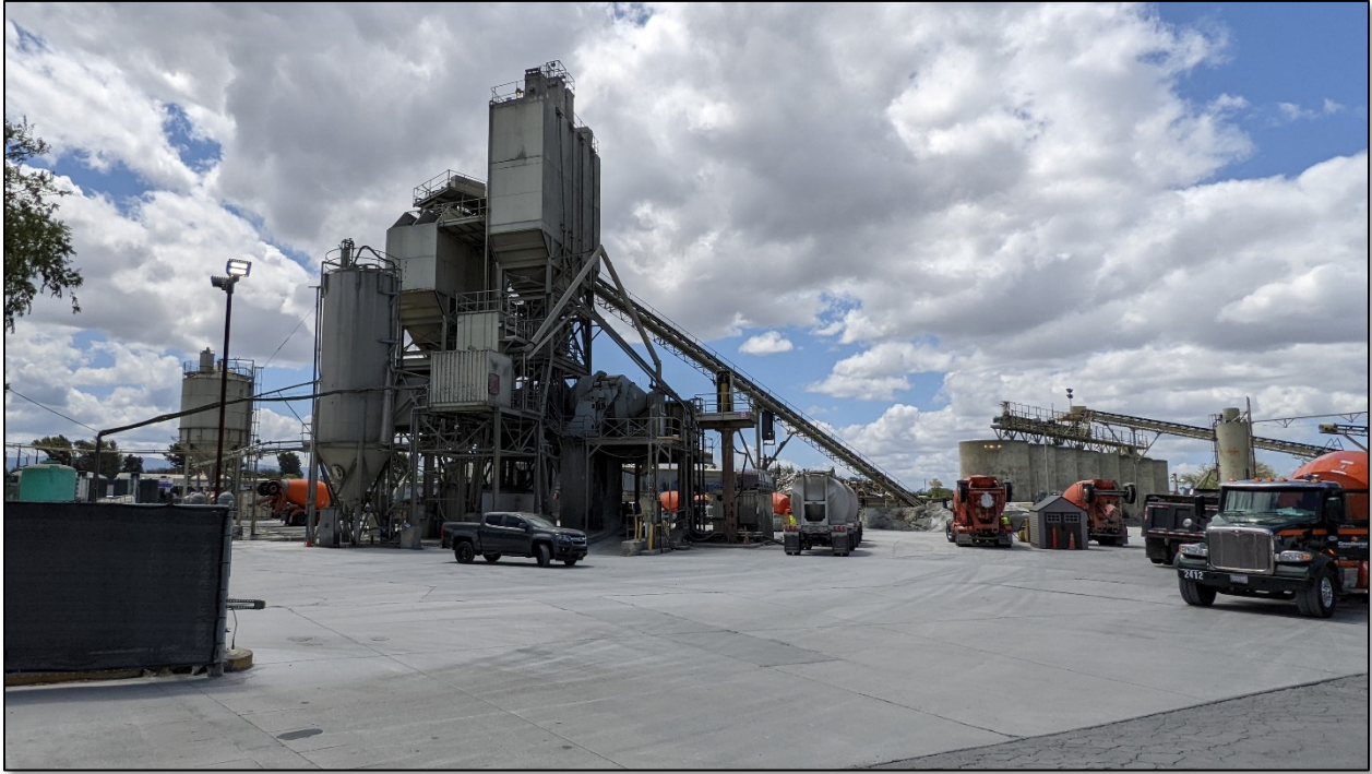
View of the concrete operation located on the subject property, as seen from near the Berryessa Road frontage
