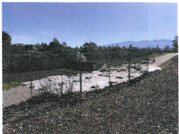
Fencing around sinkhole - failing outfall
