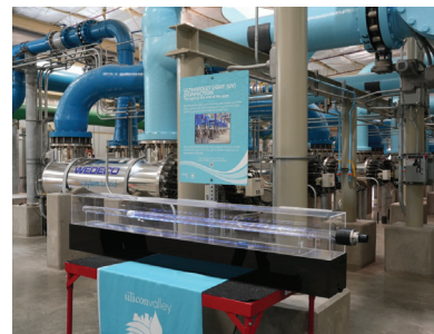
Example of a learning exhibit at the Silicon Valley Advanced Water Purification Center.
