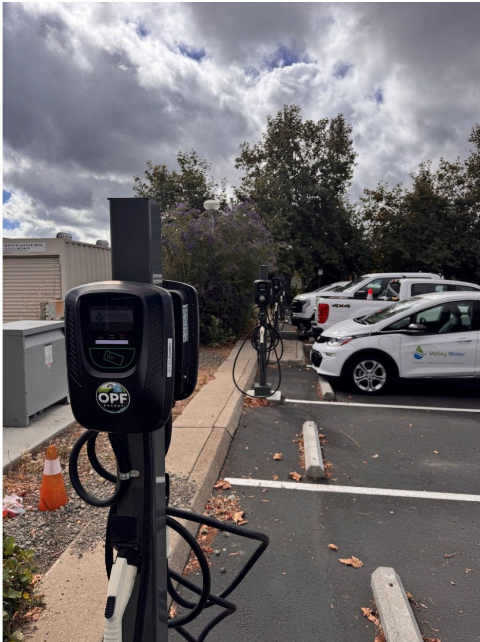
Figure 2-10. Existing Fleet Level 2 EV Charger
