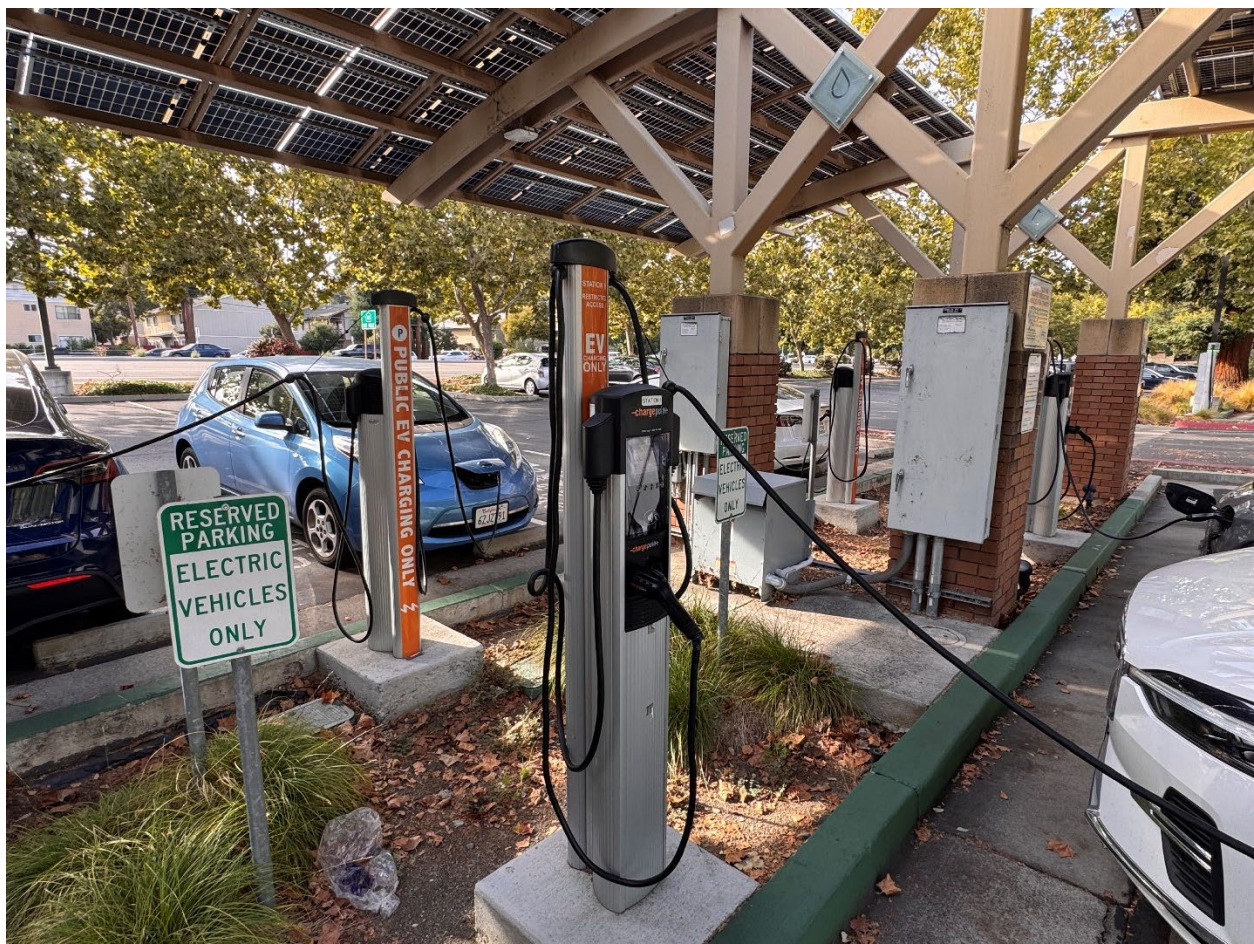
Figure 2-9. Existing Staff and Public Level 2 EV Charger
