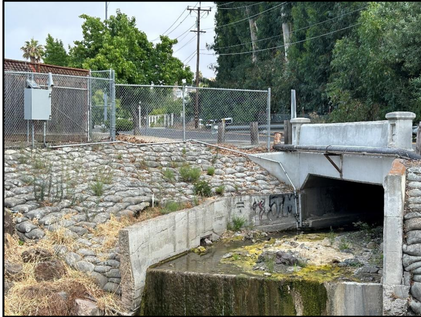
Reach 12 – Looking upstream at the Old Piedmont Road culvert and drop/grade control structure with ALERT stream gauge
