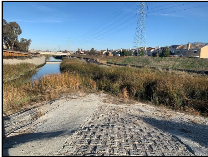
Reach 1 – Looking Downstream at Lower Penitencia Creek confluence with Berryessa Creek and levee on right
