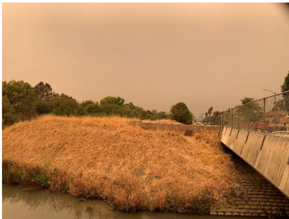
Looking west down floodwall and levee at Cunningham Avenue (culvert on right)
