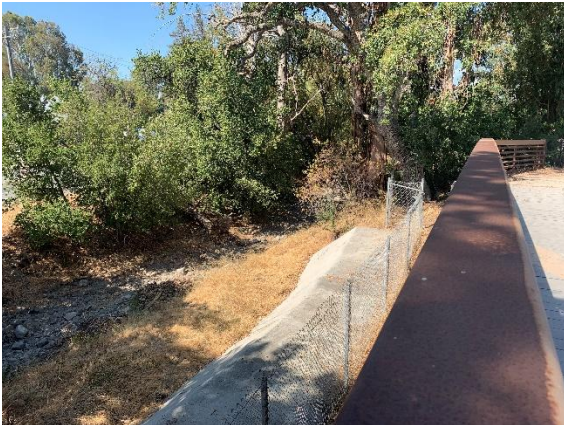
Pond overflow to creek at Bob Gross Ponds.
