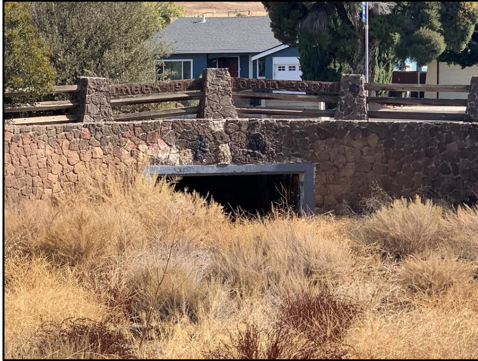
Reach 12 – Looking from downstream of Piedmont Road at exit of approximately 400-foot culvert that crosses under Cropley Road and Piedmont Road.
