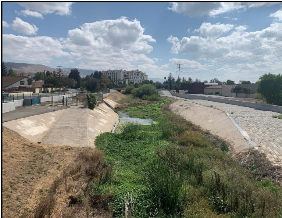
Reach 3 – Looking upstream from pedestrian bridge at north levee (left), south floodwall (right), confluence with Tularcitos Creek (on left), and Hetch-Hetchy crossing
