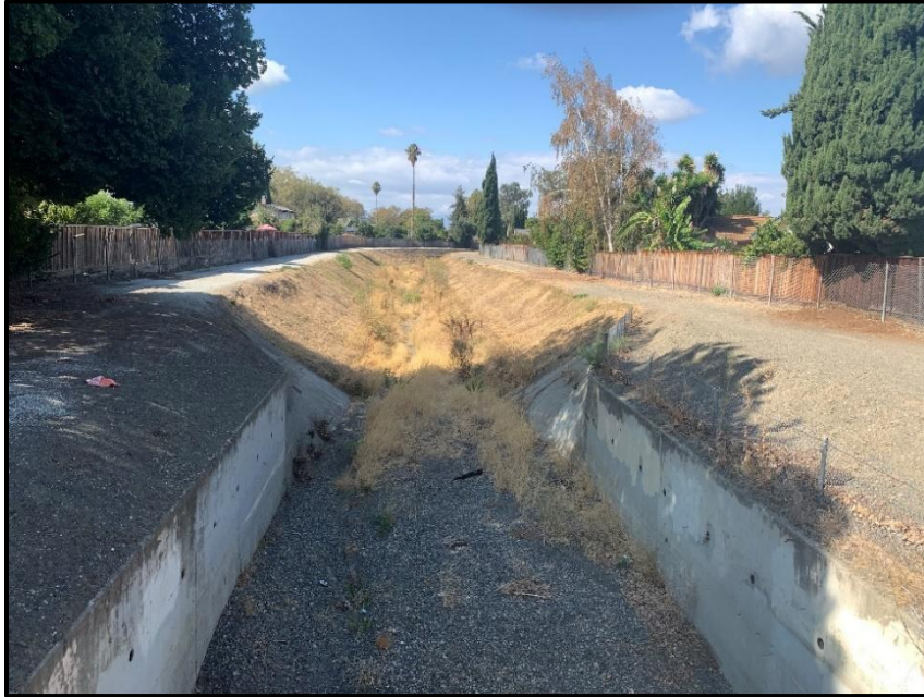
Reach 9 – Looking downstream from Morrill Avenue at concrete transition to excavated earth channel
