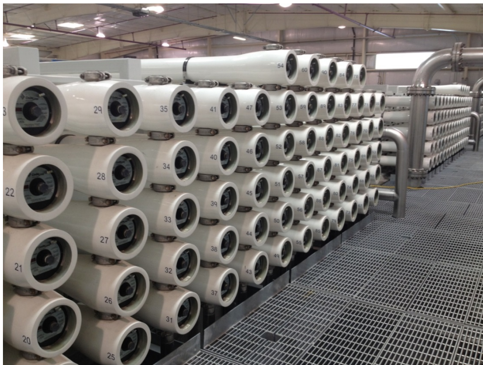
Figure 6-7: RO System at the Existing SVAWPC
